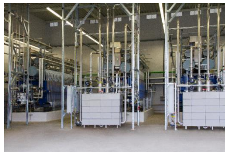
Electrolysis of the AUDI PtG plant in Werlte, Germany
