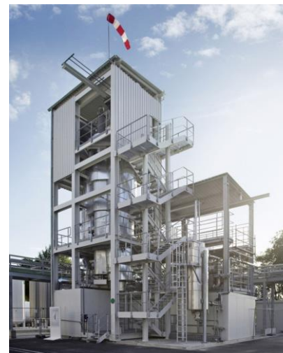
Methanation of the AUDI PtG plant in Werlte, Germany
